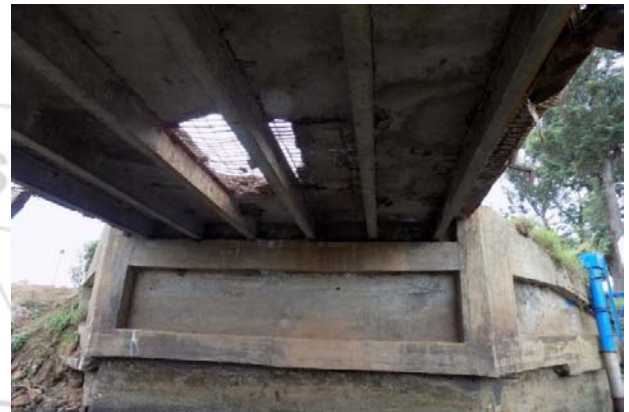
Figure 14: Falling off of the plastered underside of the superstructure slab aimed at concealing the exposed reinforcement bars
