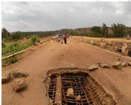
Figure 7: Manafwa River Bridge superstructure cross section immediately after the failure and before the visual inspection on the bridge (L-R).
