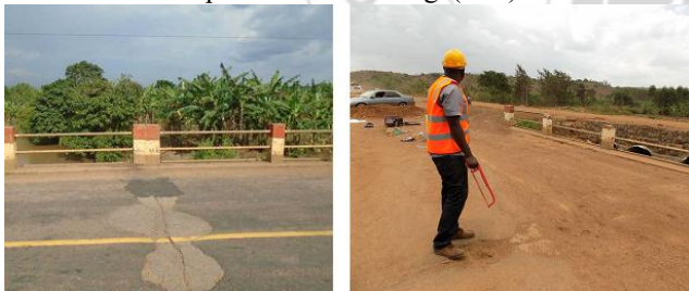
Figure 8: Transverse crack in deck surfacing and concrete patching. There is no transverse joint in the concrete slab on the underside
