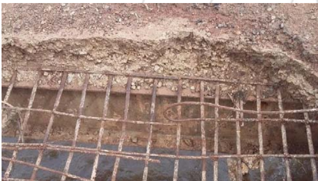
Figure 2: No hogging reinforcement in the slab, the concrete looks generally weak with a higher percentage of coarse materials
