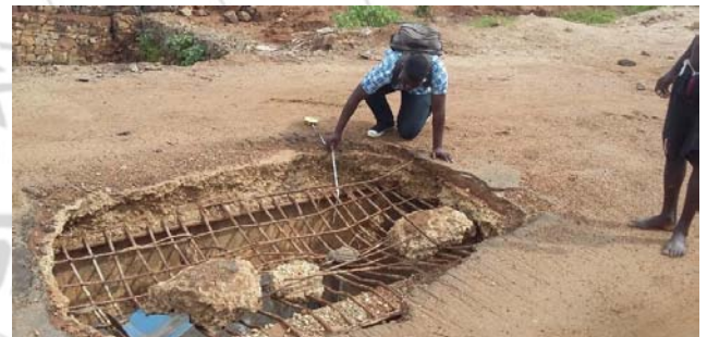
Figure 12: Bottom reinforcement at failed slab location. The reinforcement is diameter 16mm round bars at 100mm centres
