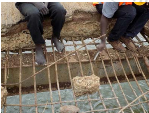
Figure 3: The longitudinal steel beams appear to have no shear connectors
