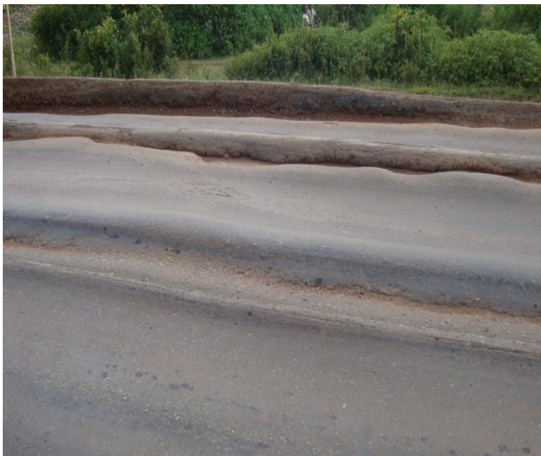
Plate 1: Severe rutting observed along the road section
