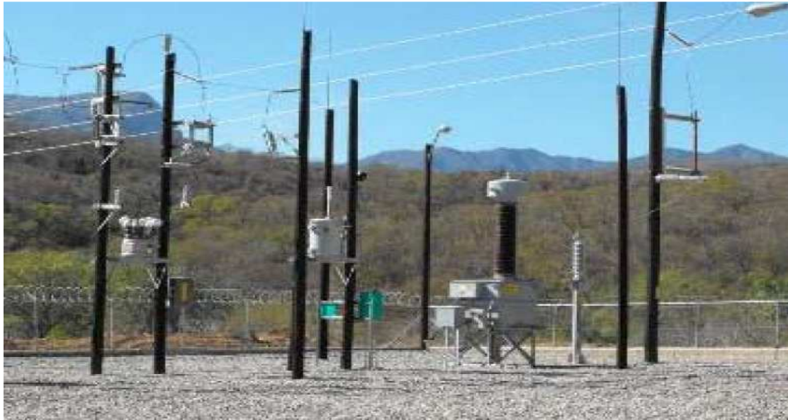
Figure 2. Auxiliary service voltage transformer (ASVT)
